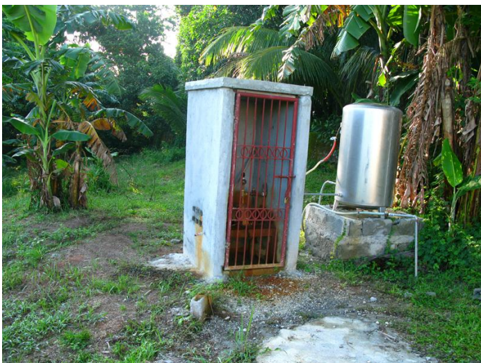
This is the well pump house and pressure tank
